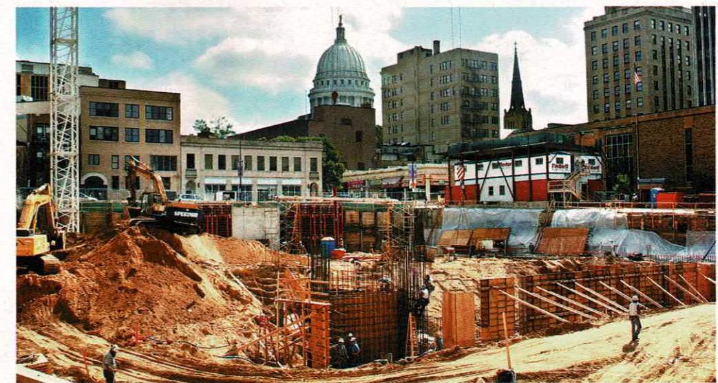
JULY 2001: Taken from Henry Street, this photo shows the Madison Public Library, 201 W. Mifflin St.
