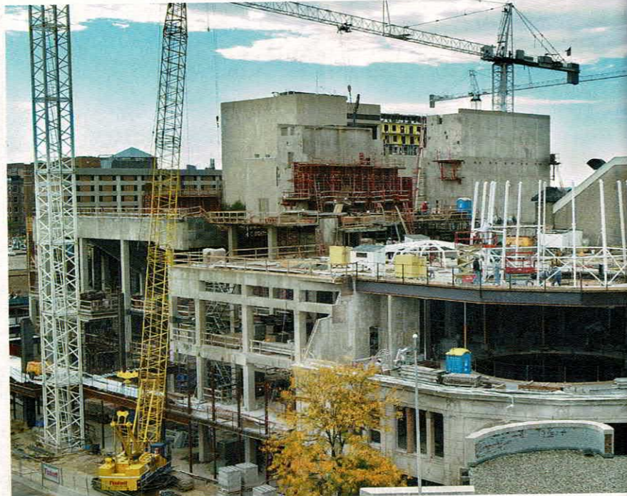
OCTOBER 2002: A construction crew works to secure the "legs" that will support the glass dome over the Overture Center for the Arts' main entrance.
